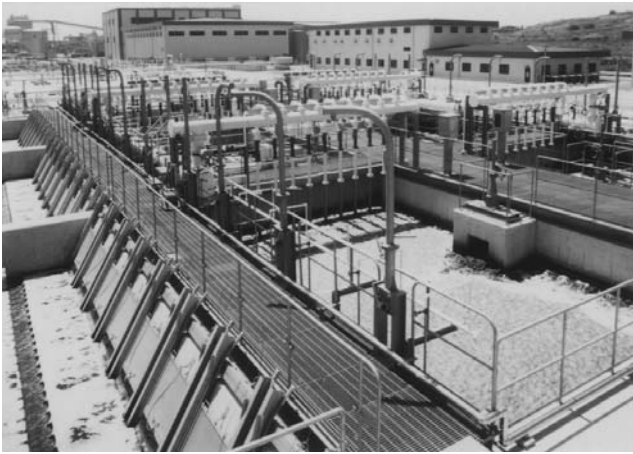
Figure 9. Photograph of denitrification plant using charged photo-cross-linked resin gels in Tokyo. Nitrifying tank volume, 10,000 m 3 , Packing ratio of gel, 10%.
